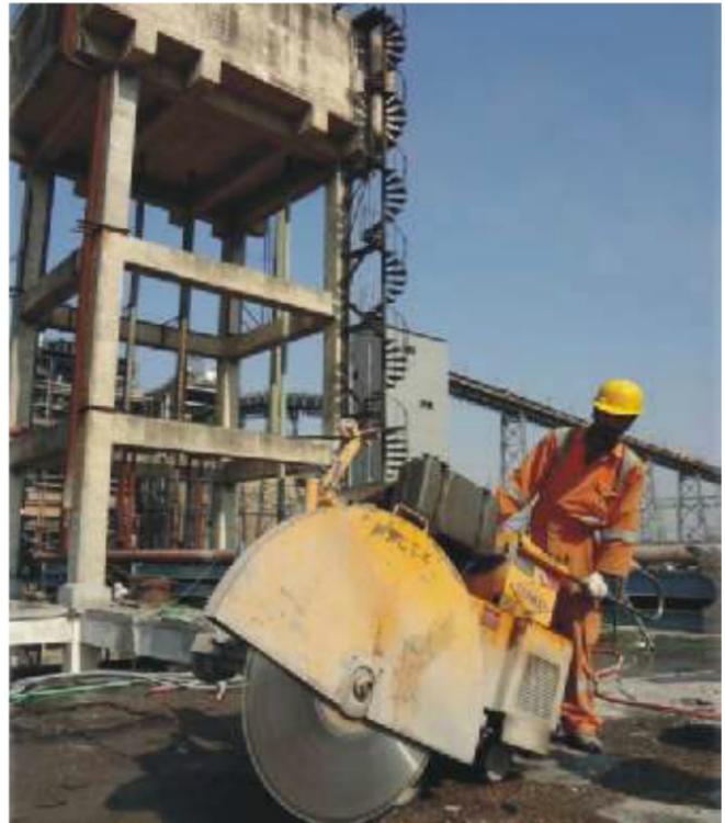
Floor sawing in progress showing the View of over head water tank to be retained After demolition of dm plant
