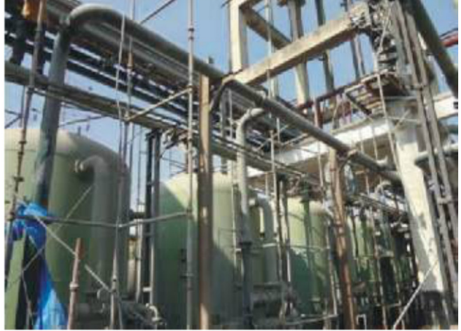
Pic showing part of Veseels and Pipe Line Arrangements below cutting area
