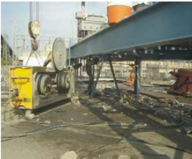
Wire Sawing of RCC Slab showing the complexity of cutting due to many pipes running in the cutting area
